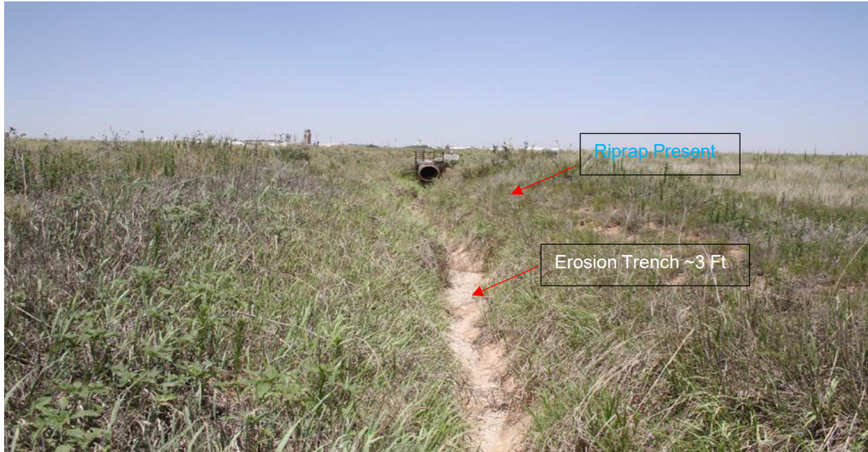
Photo 2-13. Culvert 5 and Erosion Trench
