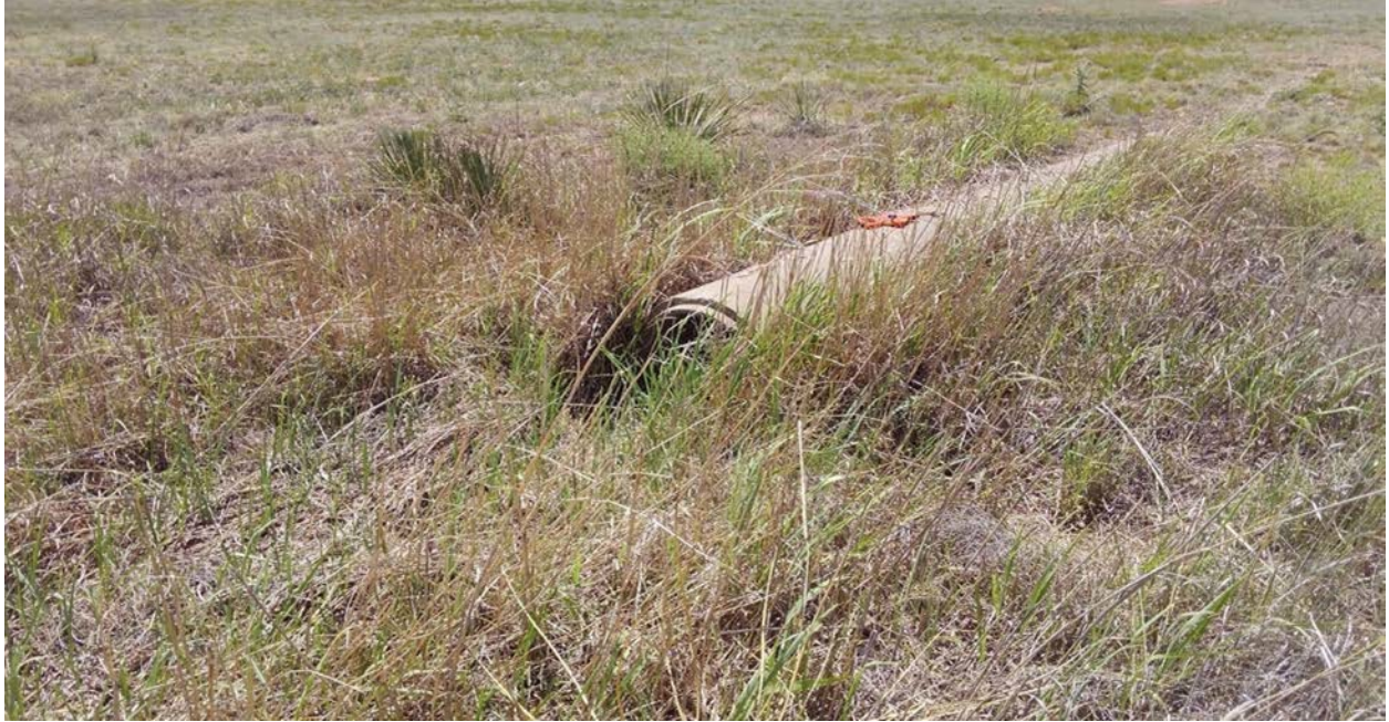
Photo 2-7. Erosion Trench at Culvert 2
