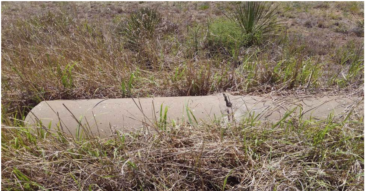
Photo 2-8. Separation in the Stormwater Line at Culvert 2
