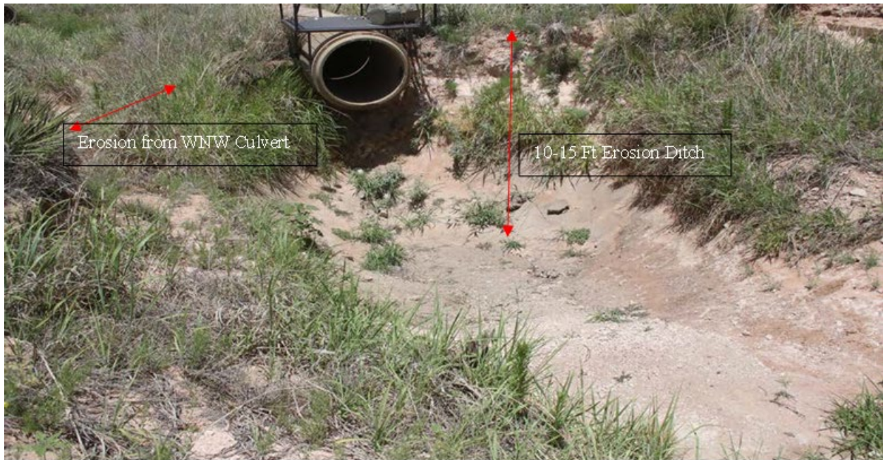
Photo 2-12. Erosion Around and Beneath Culvert 5
