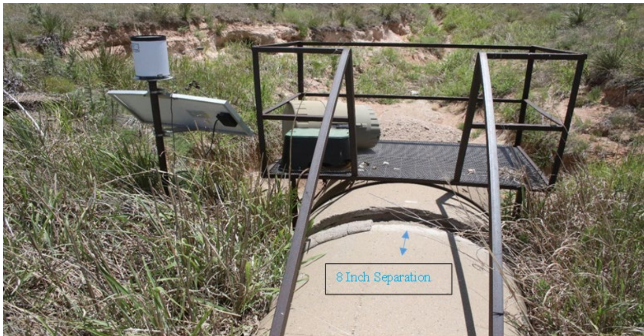
Photo 2-14. Separation in Culvert 5 Stormwater Line
