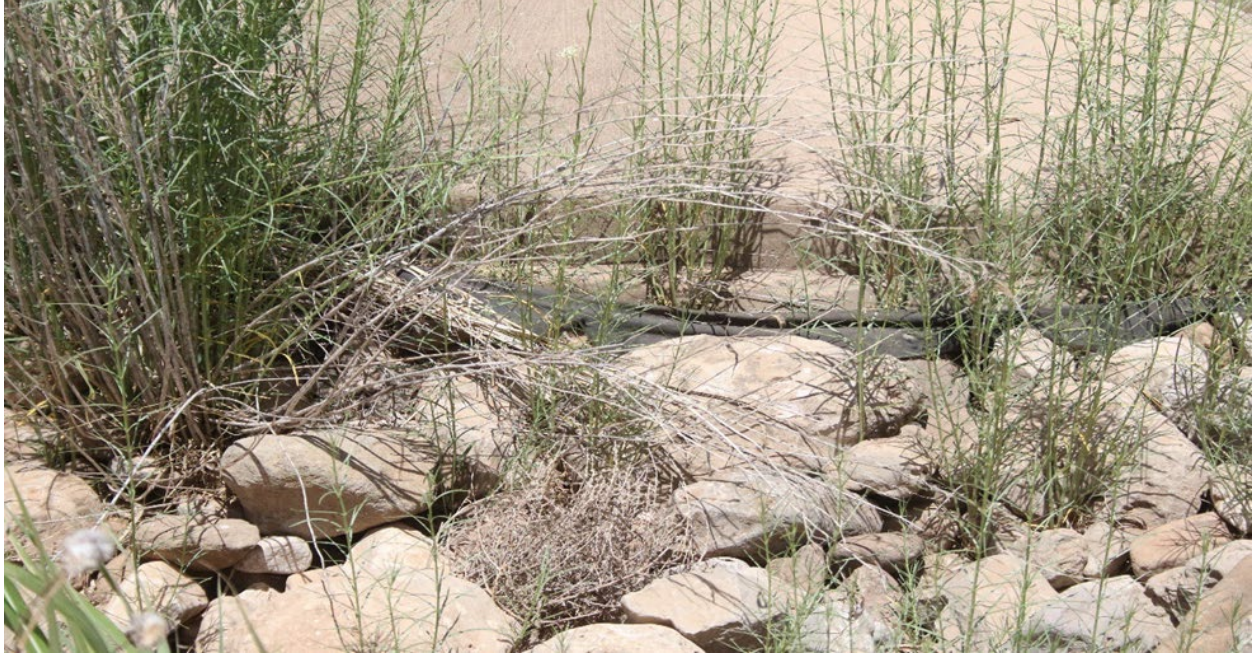
Photo 2-5. Washed-Out Riprap at Culvert 1
